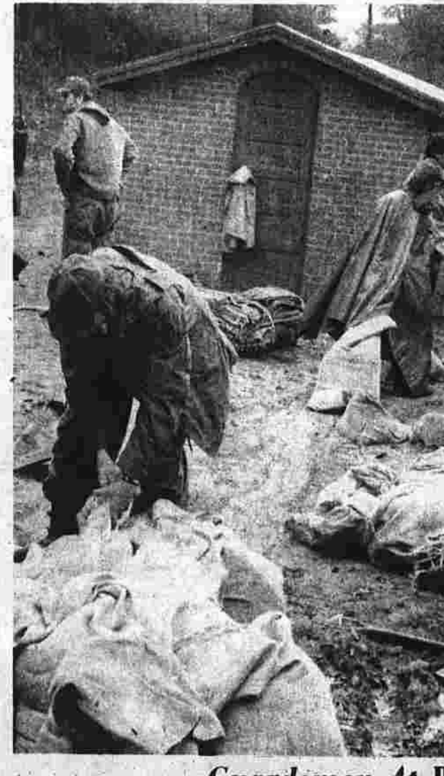
National Guardsmen fill sandbags to bolster the Lydall Reservoir Dam, which at one point Friday afternoon threatened to burst and unleash tons of water in the northeast section of Manchester. Guardsmen filled about 25,000 sandbags and saved the dam. (Herald photo by Pinto)
